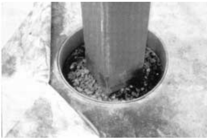
Fig. 9 – Column round isolation section not located at construction joints. Note: soft polyethylene foam isolation joint material (instead of stiff premolded joint filler used for typical PCC floors) to allow for SCC movement; peeled back special curling sheets of white, synthetic fiber with white plastic backing.
