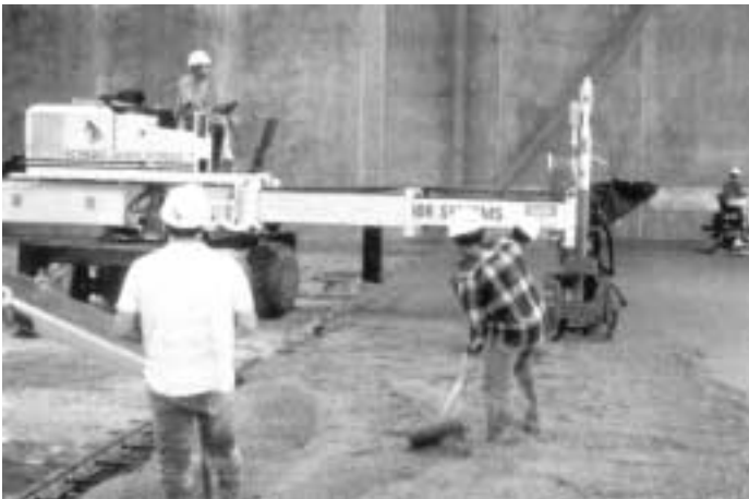
Fig. 7 – Laser screed striking off and consolidating concrete placement by means of telescoping boom with elevation controlled by laser. Laser screed assisted in attaining high (thus good) FL (levelness) numbers. Note: optimized concrete mixture that appears harsh and “stony” but is actually extremely workable and finishable.
