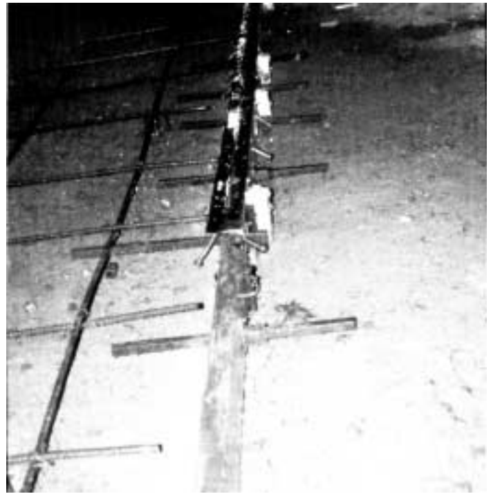
Fig. 3 – Prefabricated system consisting of steel angle armored floor construction joint, edge forms with and without armor angles, reusable dowel holders/aligners (red), etc. Note: No. 4 (12 mm) reinforcing steel at 18 in. (450 mm) on center for proper SCC expansion restraint, not structural purposes.
