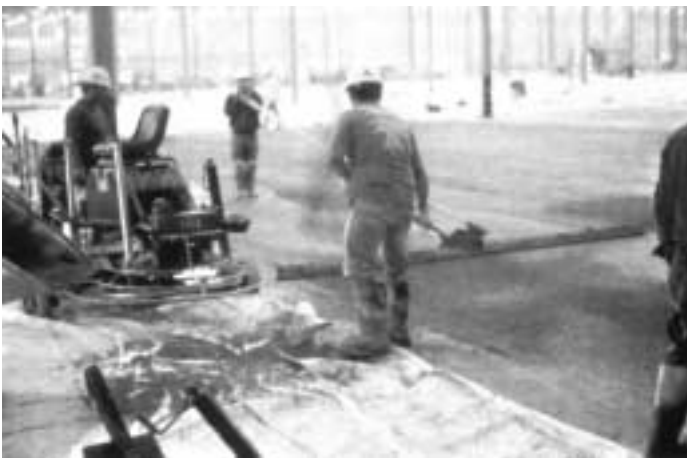
Fig. 8 – SCC floor finishing and application of field-mixed trap rock hardener. Note: 12 ft (3.7 m) long highway straight-edge assisted in attaining high (thus good) FF (flatness) numbers. Note: riding double-towel machine at left, which also helped in attaining a very flat floor when “pizza pans” were attached to the blades.
