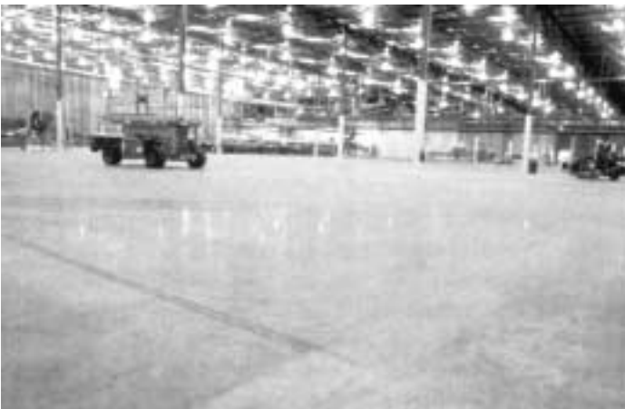
Fig. 10 – SCC finished floor with joints as far apart as 125 ft. (38 m). Note: steel angle armored construction joint (extending from center to left of photo) in lift truck traffic aisle; tight floor joints exhibiting very little shrinkage, considering large slab panels.
