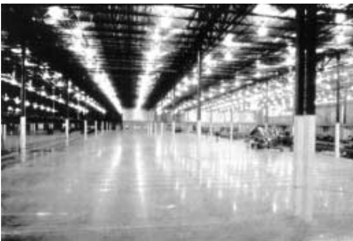
Fig. 11 – Finished slab with as much as 125 ft (38 m) between joints. Note: very straight column reflections, indicating a very flat floor; shiny, burnished floor surface (there is no coating or sealer causing the shine); armored angle construction joint in foreground.
