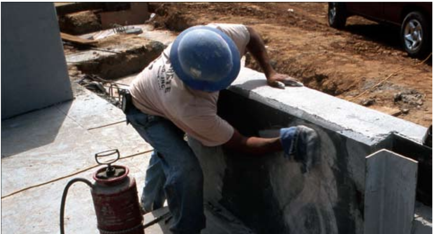
Old methods of sacking and patching required laborious rubbing and meant visual uniformity of results could be difficult. After wetting the wall with a cement slurry, laborers had to rough a silica sand/cement mixture against the wall and rub it into the surface.
