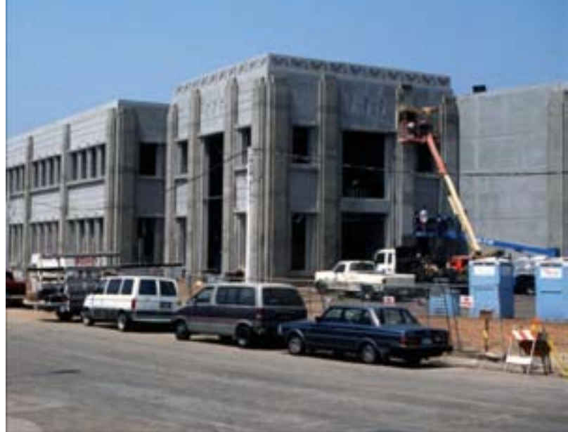
A Santa Fe, California, tilt-up concrete warehouse project comprising a two-story office and a high-bay structure relied on the abilities of new patching compounds to ensure a smooth finish.
